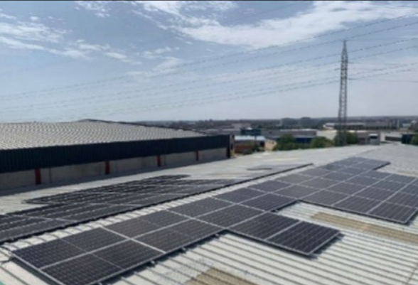
Solar panels at Intersurgical Spain
